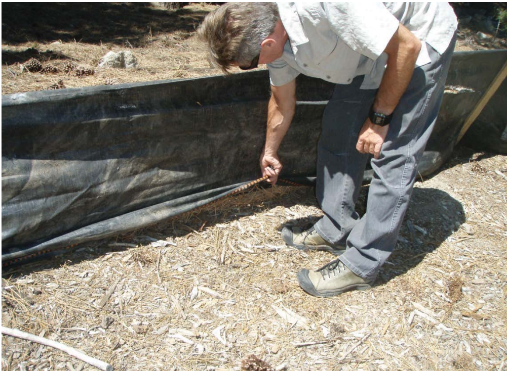
This silt fence needs to be keyed into the soil properly.
